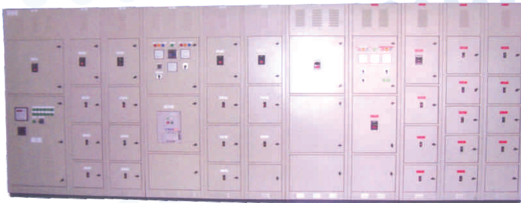
L.V. Main Switchboard with Emergency Main Switchboard (Form 3 & 4)
