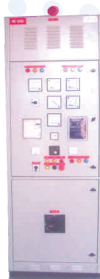
AMF PANEL SWITCHBOARD (Form 3 & 4)
