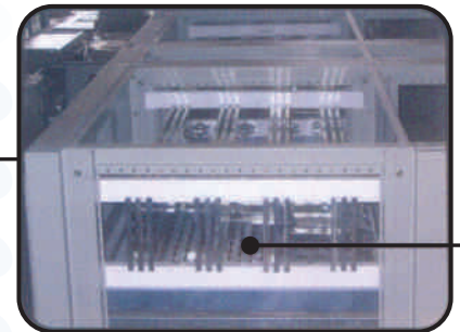
Horizontal Busbar Compartment
